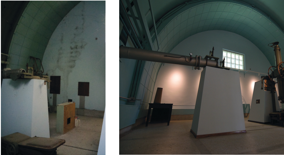
Figure 2: Photographs of the Large Transit Instrument: before remediation - left panel; after remediation - right panel.
