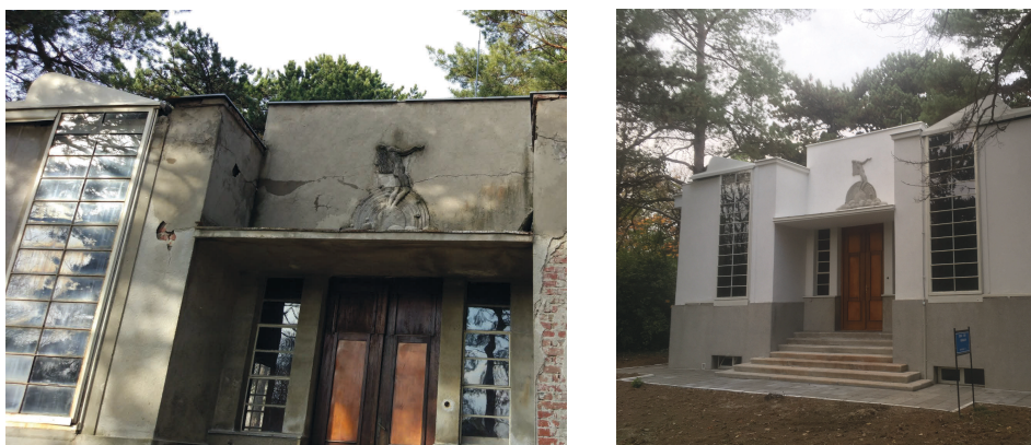
Figure 5: Photographs of the School Pavilion: before remediation - left panel; after remediation - right panel.
